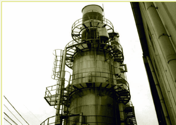
Flue gas stack from boiler fitted with economiser
